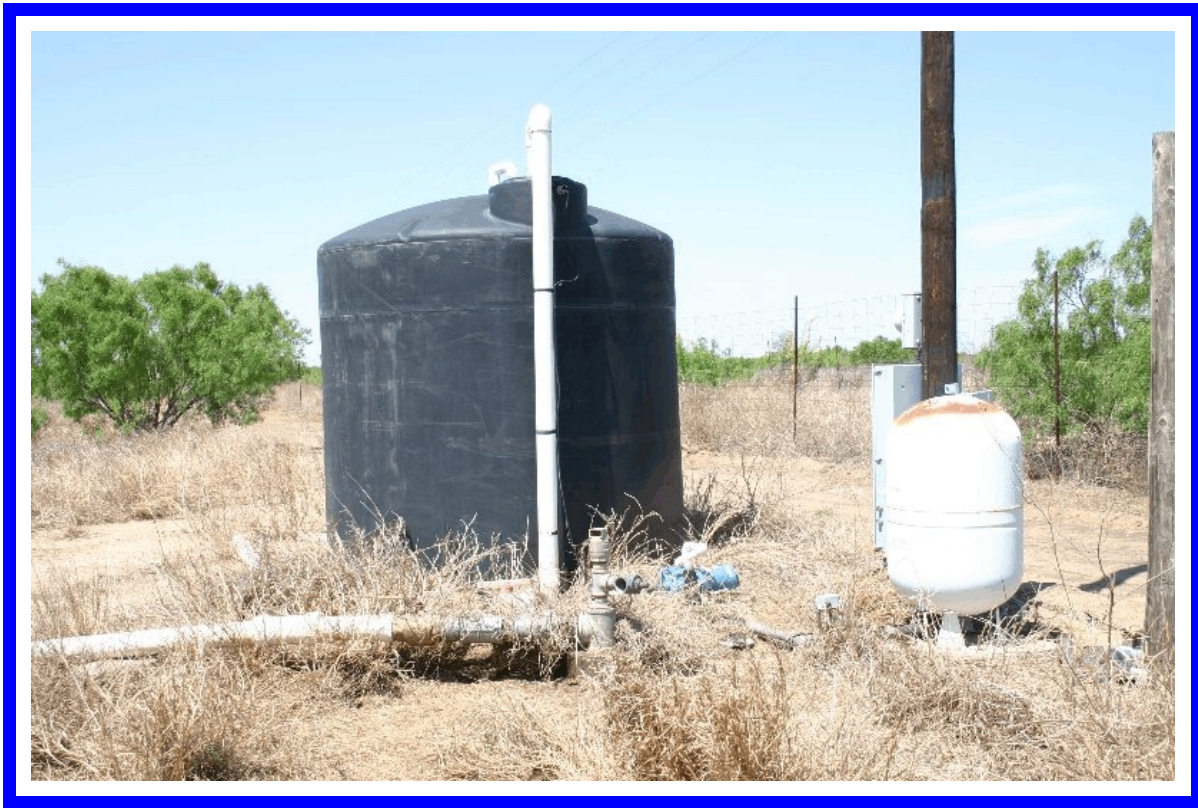
VIEW OF WATER WELL
